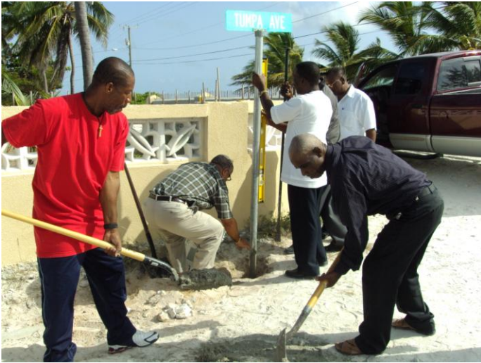
Members of the Native Men's Fellowship mixing cement and planting the street sign.
